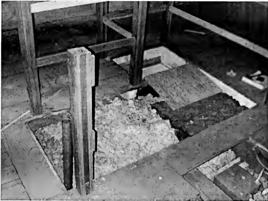
Figure 39 Third generation Stair Opening in Attic of Center Section of the Main House, 2002
